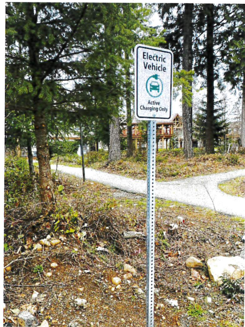
Right: multiple charging stations for electric vehicles have been installed at the Comox Valley campus.
